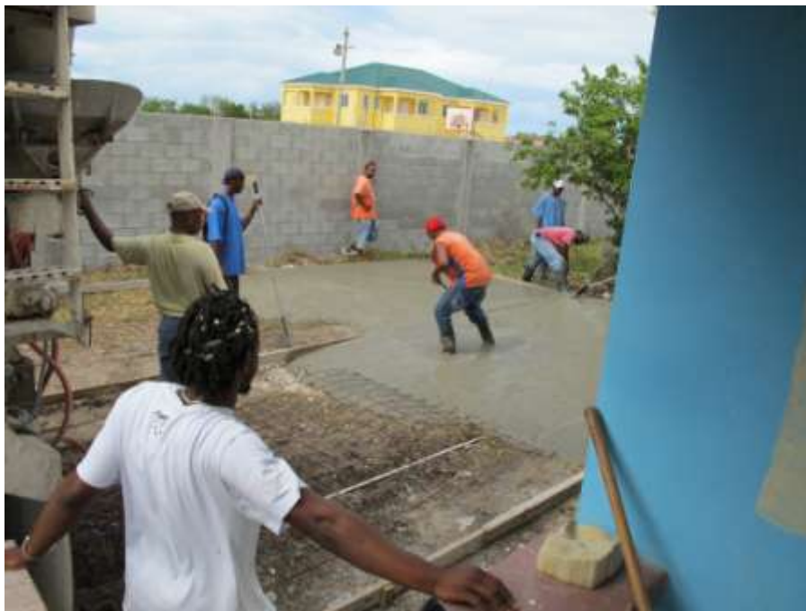
Figure 14. Barbuda Council crews pour cement slab around the Research Station Main Building. The concrete was donated by a local contractor and the labor was provided by the Barbuda Council and the High School Manual Arts class. The concrete surface will be covered with shade structures to provide outdoor classroom and wet lab working space.
